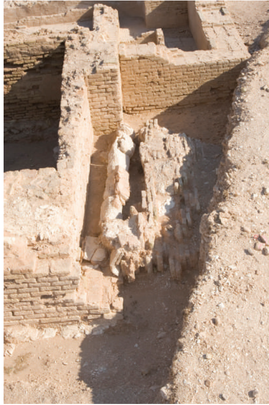
Figure 1.19 View showing collapsed exterior wall at south-east corner, which was not in bond with the interior wall.
