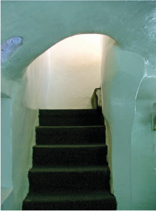
Figure 3.49 Crypt, staircase with uneven wall masonry and blind window-like structure on top left. Photo: Author
